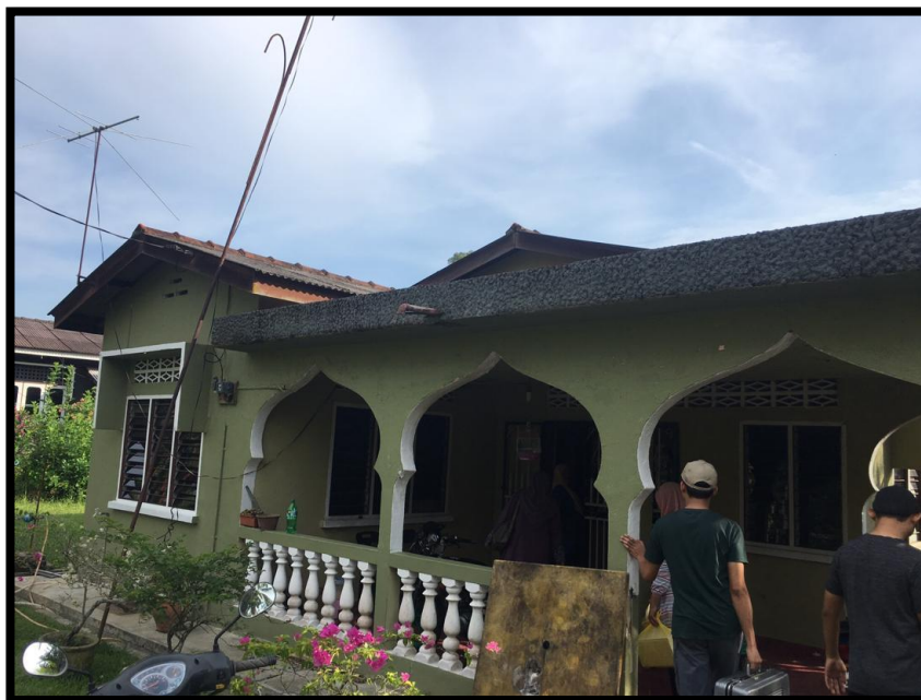
Figure 13: Houses with asbestos roofing
